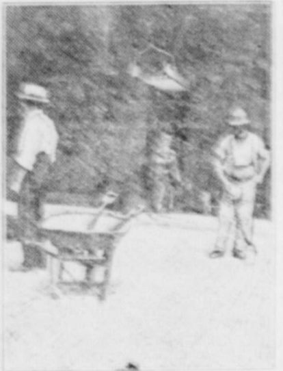
Grading Blocks Laid and Ramped—Maintenance Cost of This Kind of Roadway is Less Than That of Any Other Kind.
