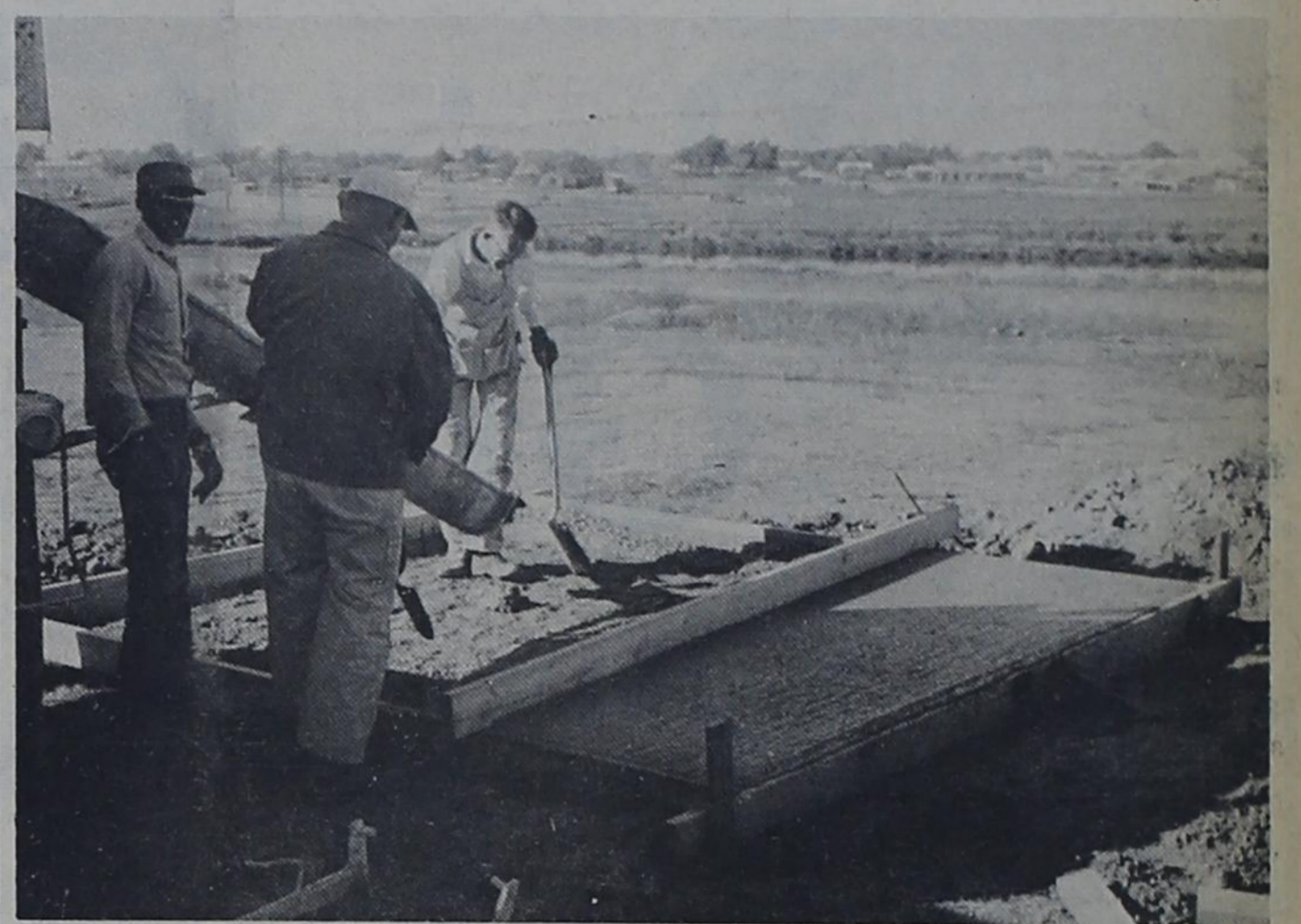
CABLE TV GROUNDWORK -- Foundation for a building to house electronic equipment connected with new cable TV system was being poured here this week. Arnold Hroma, right, and Lawrence Gray, center, were working with the project. The tower for the system is to be erected in city dumpgrounds on east side of Bovina with the building to be located near it.
