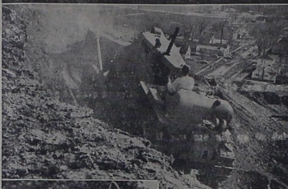
GOUGING FOOTHOLD on side of mine waste pile above Wenona, Ill., D8 prepares site for emergency warning radar station. (CNS PHOTO)
