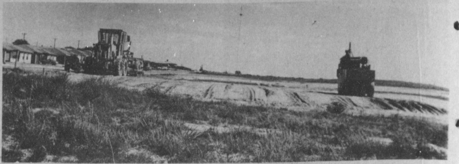
DIRT WORK STARTED.... Heavy equipment has been moved to the location of the senior citizen housing complex on West Avenue K. Dirt work has started this week and construction is expected to begin in the near future on the first 20 units of the controlled rent housing. Senior citizens are the only persons who will be allowed to reside in the new housing. Also, an additional 30 units will be applied for as soon as construction on the initial phase gets underway.
