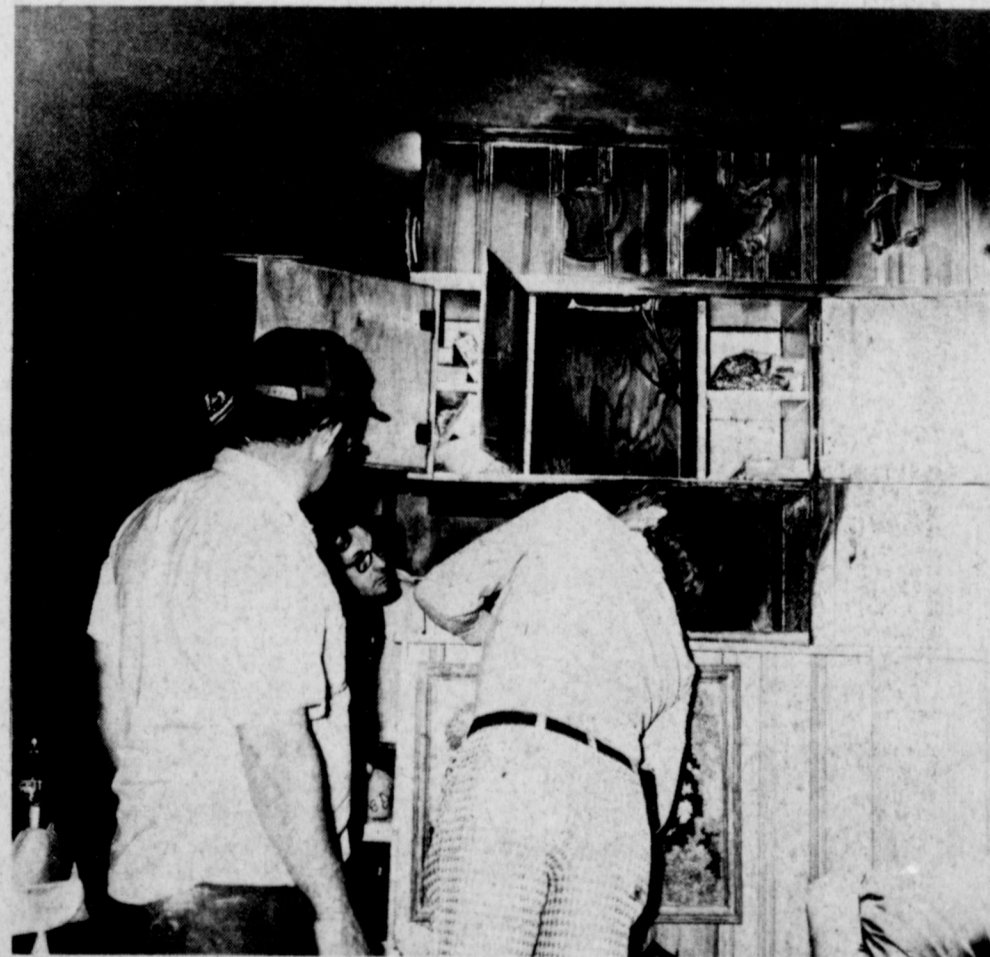
FIRE AT SHAW HOME... Mrs. Eugene Shaw returned to her home on FM 1760 Thursday afternoon to find her kitchen blazing. Damage was sustained by the kitchen and den areas of the home from a suspected electrical fire originating above a cabinet. Here, members of the Muleshoe Fire Department check for smoldering wood after extinguishing the fire.
