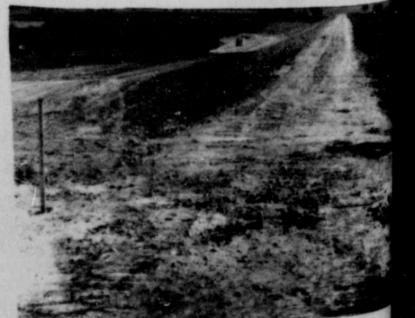
View of top of completed dam and start of construction of fence looking east.
