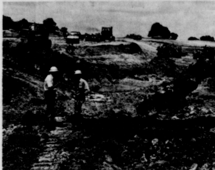
A core trench is dug and back filled with good clay to cut off sweep water. Mills
