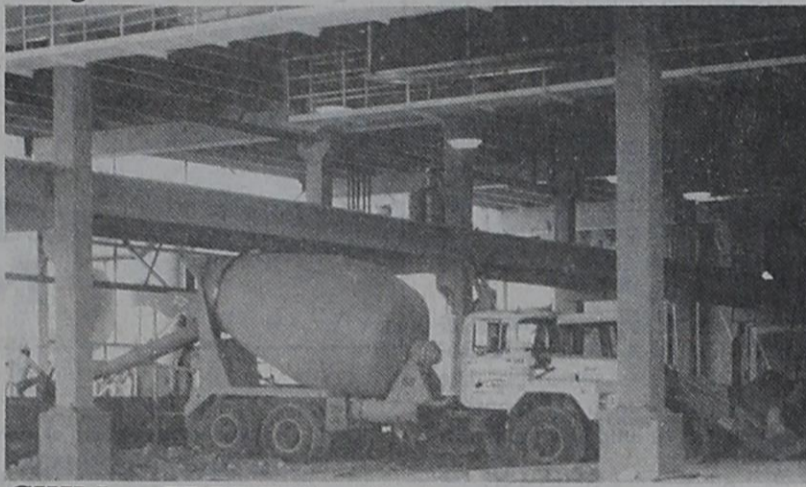
CHILL FREEZER... Workers are shown pouring concrete at the site of the new chill freezer being built at Excel. The facility will double the freezer capacity.
