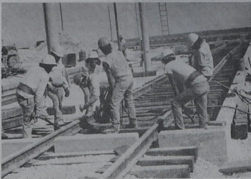
RELOCATING TRACKS... The railroad tracks, located behind Excel, had to be completely uprooted and moved in order to make room for the new expansion. Workers are shown taking advantage of the good weather.
