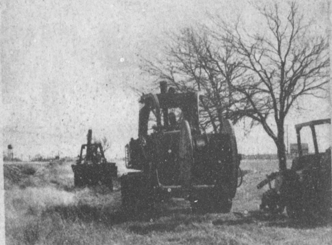
GTE TOLL CABLE--Construction is underway in placing 34 miles of toll cable between Littlefield and Muleshoe, to be used for handling expected increases in long distance service over the next 10 years. Amherst and Sudan will also be provided with additional long distance and data transmission capabilities. The new facility is expected to be complete by August.
