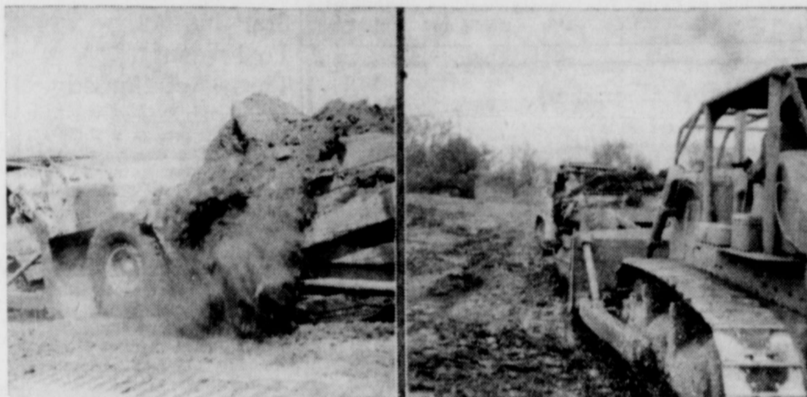
These two pictures show our machinery as used in dirt moving, building tanks or enlarging or cleaning tanks and building terraces.
