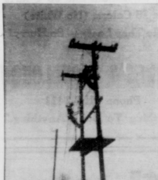
City Electricians shown installing part of Power Transformer Rack at the Off-Channel Storage Reservoir Pump Station.
