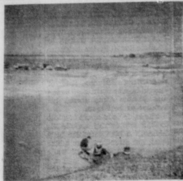
Storage Reservoir pretty well shaped up with Water caught from heavy rain. Don Blevins, Engineer, setting up Equipment to pump rainwater out so construction work may continue.
