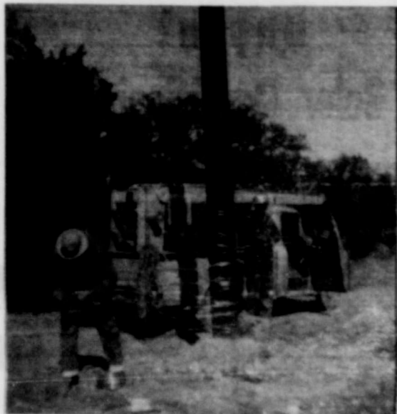
Wires being spliced by City Electricians about midway after construction of the approximately eight mile Electric Power Line.
