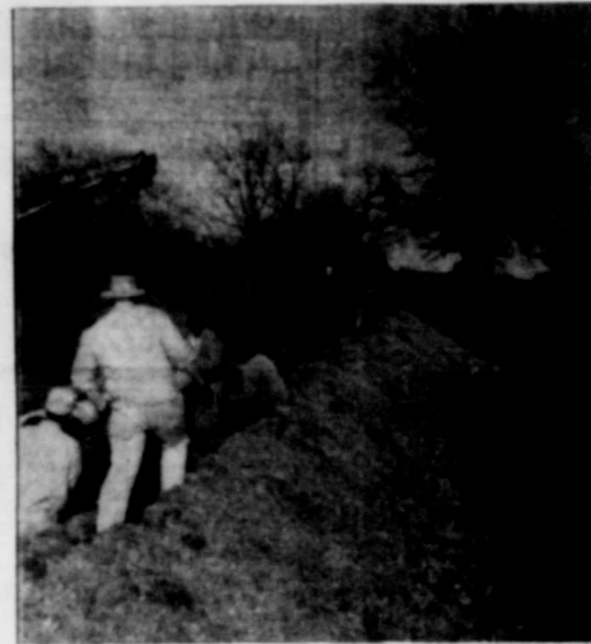
Installation of Pipeline continues across ranch country toward the Colorado River to bring adequate water supply to Goldthwaite.
