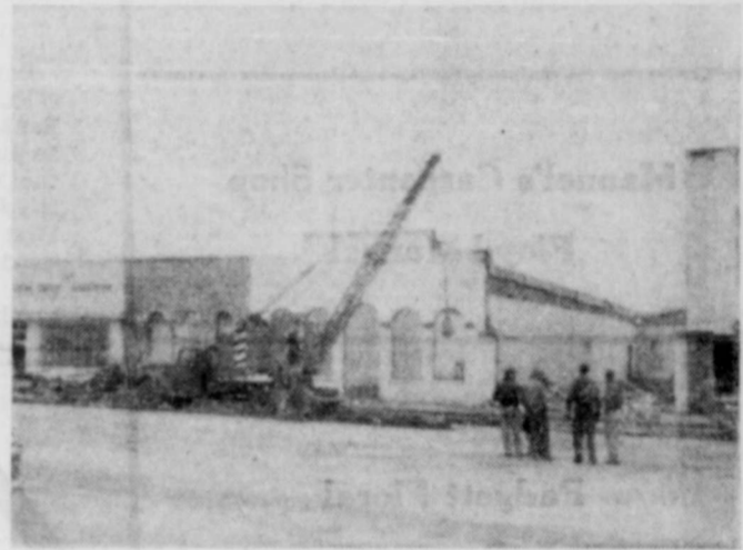
This photo shows demolition work in process. The first of three buildings had been razed and workers were moving machinery to start on the second one.
