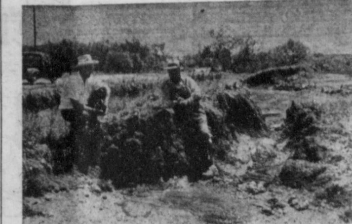
FLOOD DAMAGE —This photograph shows the damage done to a levee during recent hard rains in the Brown-Mills SCD. Runoff was too heavy during the rains and this levee gave way.
