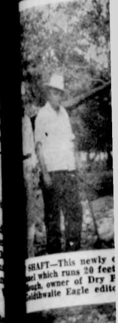
SHAW—This newly installed well runs 20 feet deep, owner of Dry E Goldthwaite Eagle edit
