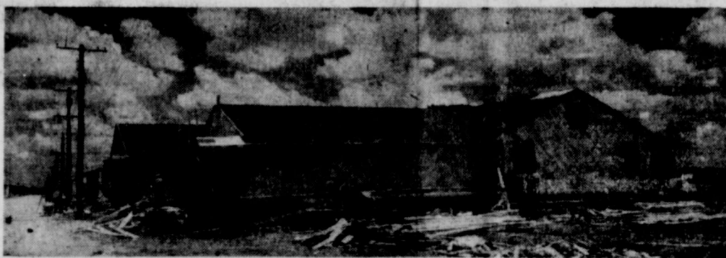
A 500-man cafeteria-style mess hall for students in the motor mechanics school at the Normoyle Quartermaster Depot at San Antonio is being constructed and is now at the half-way mark (above). Another 1,000-man mess hall is also to be erected and the two will accommodate 1,200 students at the school, which is now operating on a smaller scale. More than $1,000,000 worth of construction is under way at the Depot, according to Col. Edwin V. Dunstan, Eighth Zone Construction Quartermaster, Fort Sam Houston.—U. S. Army Signal Corps photo.
