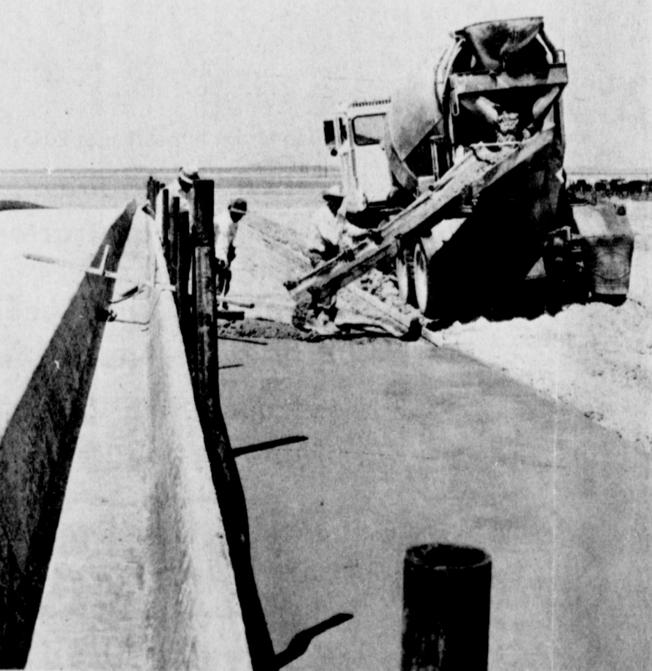
NEW FEEDLOT CONSTRUCTION--Workmen from Ready Mix Concrete are shown pouring and smoothing concrete on a standing pad at the new feedlot which is being constructed southwest of Muleshoe. Bailey County Feeders, Inc. is the name of the new facility and the owners are Jim Small, Max King and Bob Clark.
