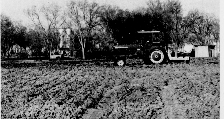
MULESHOE CITY PARK IMPROVEMENTS--Park improvement is in full swing at Muleshoe City Park in the east part of Muleshoe. City employees, utilizing donated equipment, are busy clearing, plowing and leveling the land at the park. Fry & Cox Equipment Co. is furnishing a 'Big Ox' tractor borrowed from Johnson-Nix Equipment Co. and Whitt, Watts & Rempe is furnishing a disc. Walter Barthoff, of the Muleshoe Park and Recreation Committee has said that when the park improvements are completed, there will be 35 per cent more space in the actual park than existed prior to the improvement program.
