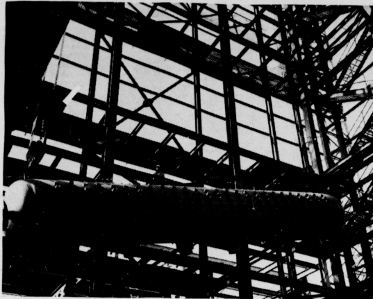
Continued construction on a 210,000 kilowatt generator at Nichols Station, northeast of Amarillo, is part of Southwestern Public Service Company's $20,000,000 improvement program for 1967. Pictured is the installation of a 225,000 pound boiler drum for the new generating unit.
