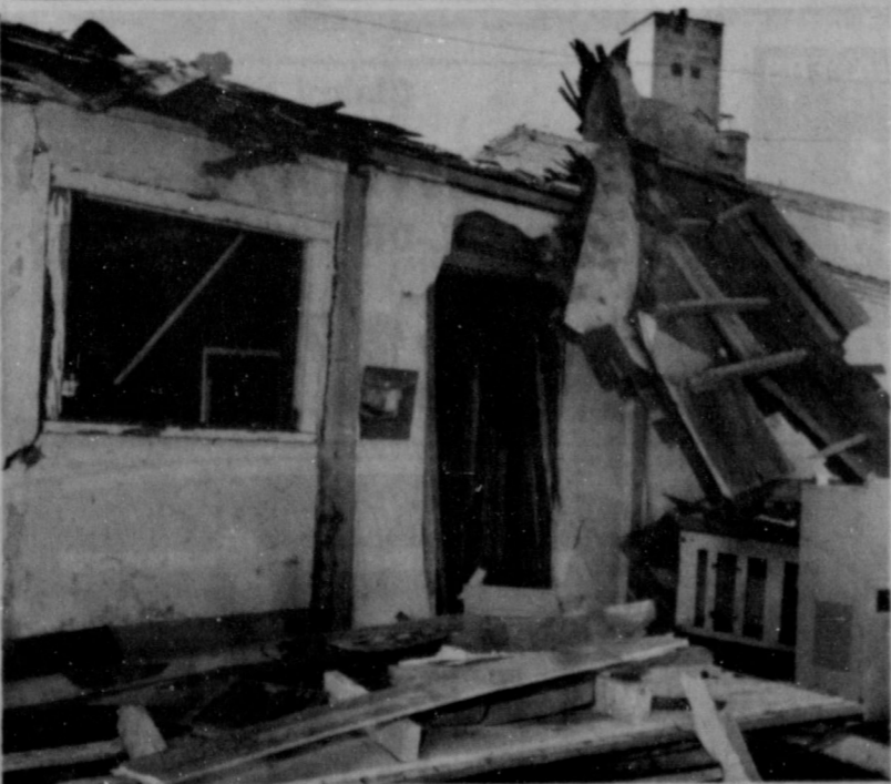
EXPLOSION--An early-morning explosion demolished a small entryway room at the office of Farmers Co-Op Gin in O'Donnell Tuesday. Above left shows debris left after the small room was leveled and a Coke box shattered. Deputy Stanley Krause and O'Donnell Fire Marshal Roger Doss decided the explosion and subsequent fire about 1:30 a.m. were accidental, possibly caused by escaping gas ignited by the Coke machine
