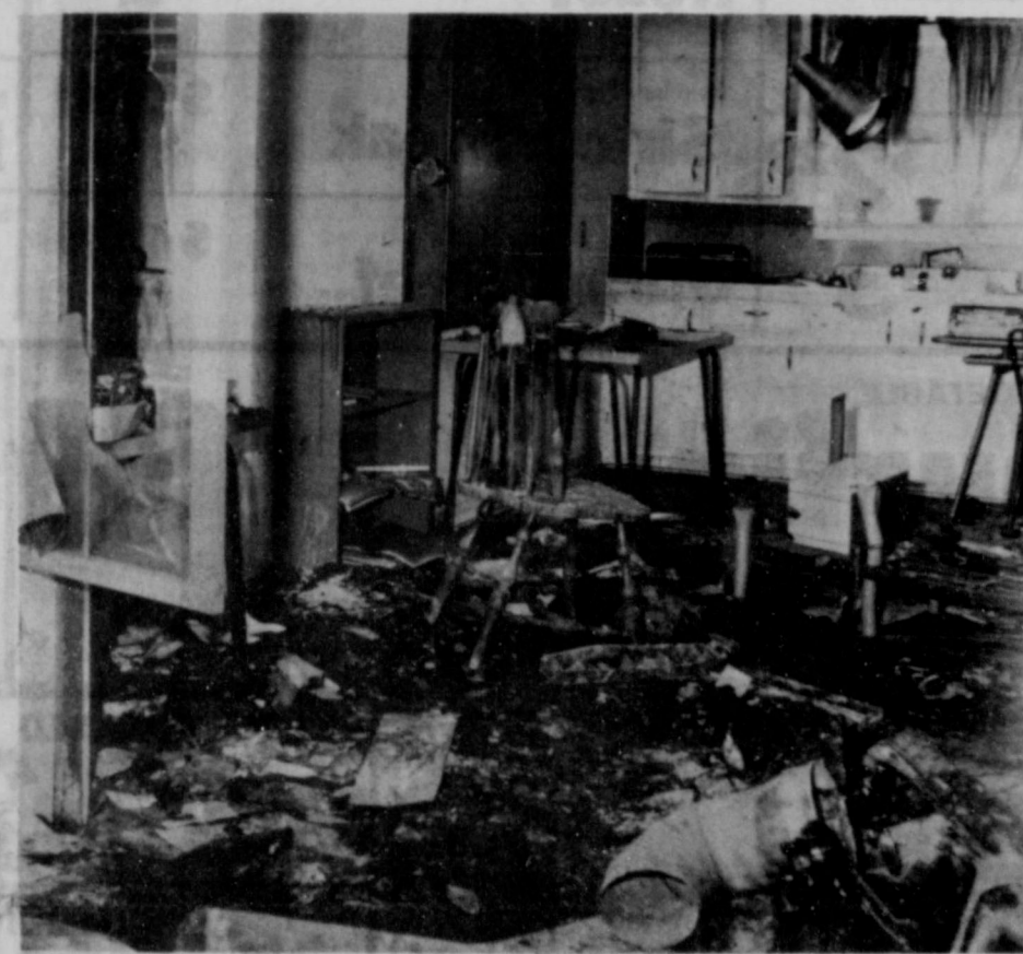
HOME EC BUILDING BURNS--Fire gutted the interior of the Tahoka High School home economics building early last Thursday. Above is some of the mess left by the blaze, caused by deteriorating electrical wiring. (LYNN COUNTY NEWS PHOTO)
