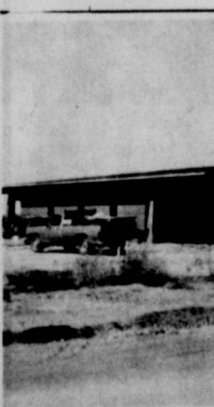
WILSON BANK PROGRESS--Construction is underway on a new Wilson State Bank building at the west edge of Wilson, and here it can be seen that the basic structure is up. Completion of the new bank is scheduled for January.
