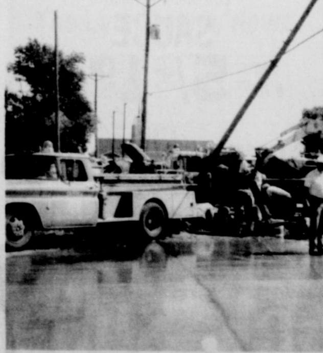
AFTER THE FLOOD - City workers spent a trying time Thursday night and most of the day Friday attempting to stop the flood of water released after a vehicle struck a fire hydrant on Lockwood Thursday night, leaving much of the city with little or no water pressure and streets all downtown with little rivers next to sidewalks. Here Police Chief Jack Miller directs traffic during the work, which had a couple of men standing in a waterhole with water up to their shoulders.
