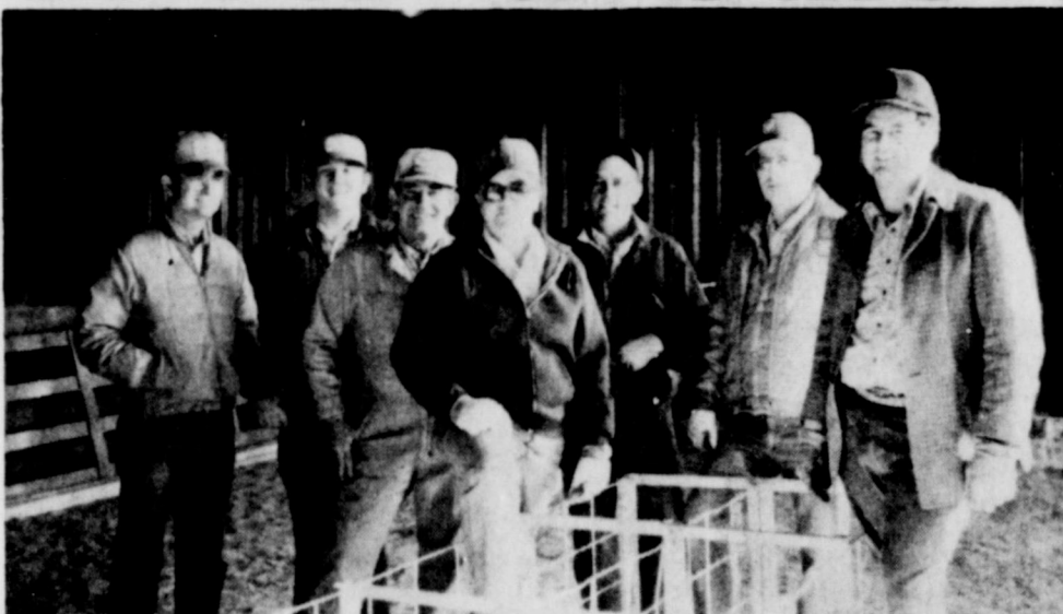
THESE MEN ARE MAKING REPAIRS and doing other work in the County Showbarn in preparation for the Lynn County Stock Show to be held there February 22-24. They revamped the sand traps in an effort to eliminate backups during the show. Those pictured but not the only ones working are: (left to right) Lyndell Wood, Tahoka, Chairman of the Building and Grounds Committee; Ray Ehlers, Wilson, Director; Cates Zant, New Home, Director; Donald Klaus, Wilson, President Elect; Jimmie Kieth, New Home, Building and Grounds Committee; Jerry Don Ross, Wilson; and Harold Sanders, O'Donnell, President of the Lynn County Stock Show Association.
