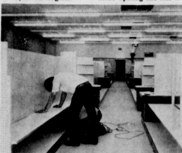
WORKERS AT THE BUILDING to be occupied by Perry's Variety Store are putting the finishing touches on a major remodeling job. The building was the former D & H Supermarket.
