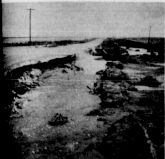
ROAD CAVES OFF - Pictured above shows Highway 10 miles south of New Moore as it was caved off by rains Sunday evening. In places the highway was cut out to the center stripes. It was reported that about 45 minutes. Photo by David Midkiff, Highway
