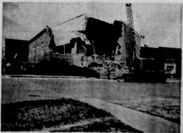
UP WITH THE NEW - DOWN WITH THE OLD - Pictured above is a picture of the New First Baptist church which will be dedicated at a later date, and the demolishing of the old church building, except for fellowship hall and a joining class rooms.
