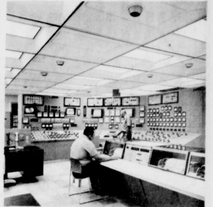
CONTROL ROOM -The control room at Southwestern Public Service Company's Jones Station, southeast of Lubbock is the terminal center for data recording equipment which takes nearly 500 readings every minute, records them and calculates their meaning insofar as plant efficiency is concerned. The plant's turbine control system is the first of its kind in the world. It utilizes a digital computer and data recording devices to bring the turbine on the line and control it during operation. Jones Station, named for Dr. Clifford B. Jones, president-emeritus of Texas Tech, will be dedicated on November 6. The plant will be open to visitors from 11 until 7 on Saturday and from 1 until 7 on Sunday, November 7.
