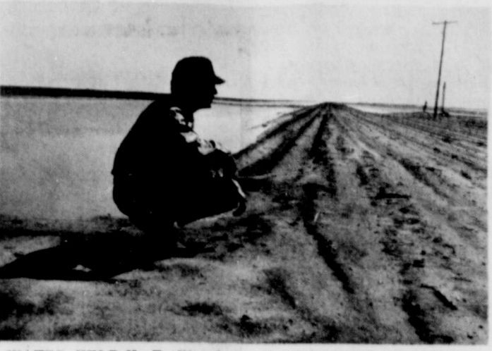
WATER HELD-K. E. Warsaw, district cooperater with the Lynn Soil and Water Conservation District looking at water held above new parallel terraces that were constructed in March and April 1971. (Photo by S.C.S.)
