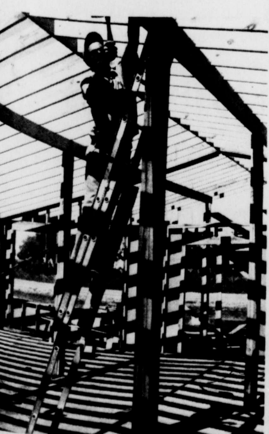
REST HOME CONSTRUCTION —The mid-morning sun Saturday gave this unusual effect to a picture of a local carpenter, Buddy Jones, as he worked on the new rest home for Crowell located southwest of the square. Construction of the new 80-bed facility is moving along rapidly.
