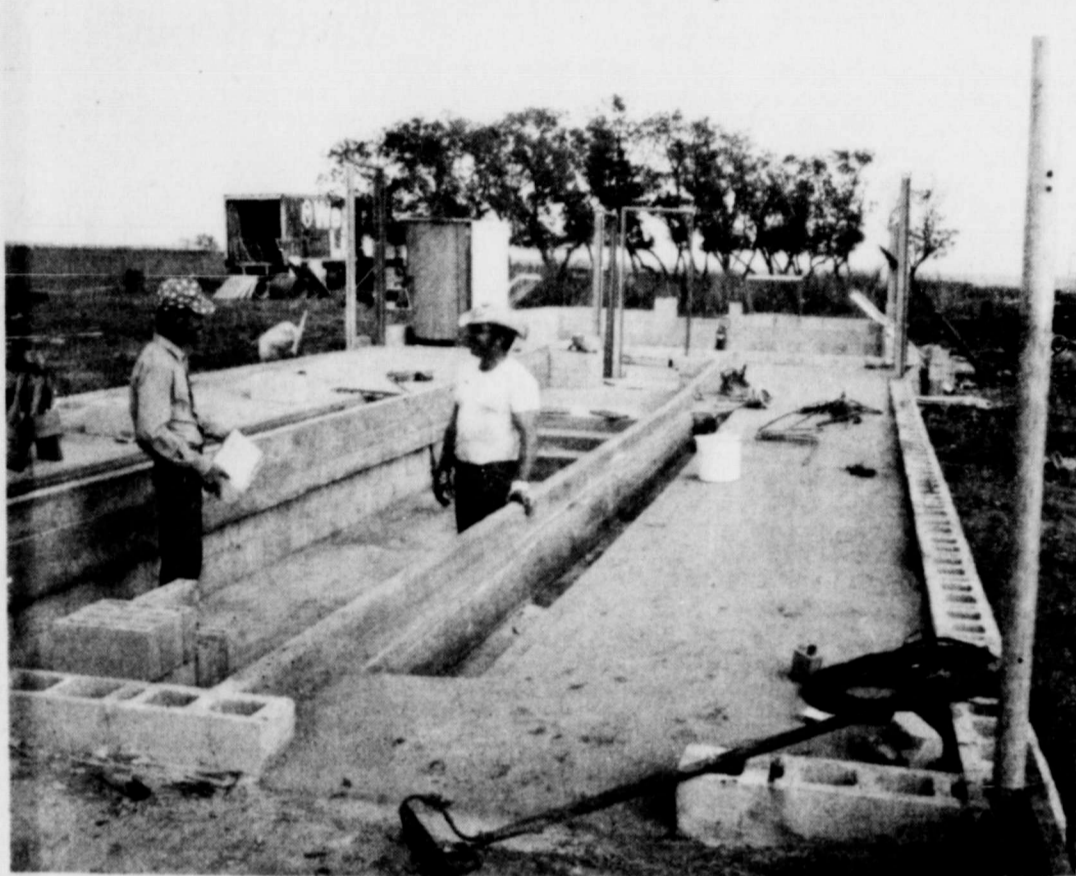
CONSTRUCTING NEW DAIRY —J. M. Parker, right, owner of a new dairy being built north of Crowell, is pictured above with Max Gerhardt as they lay concrete blocks for the building last week. The men are standing in the part of the building where the milking
