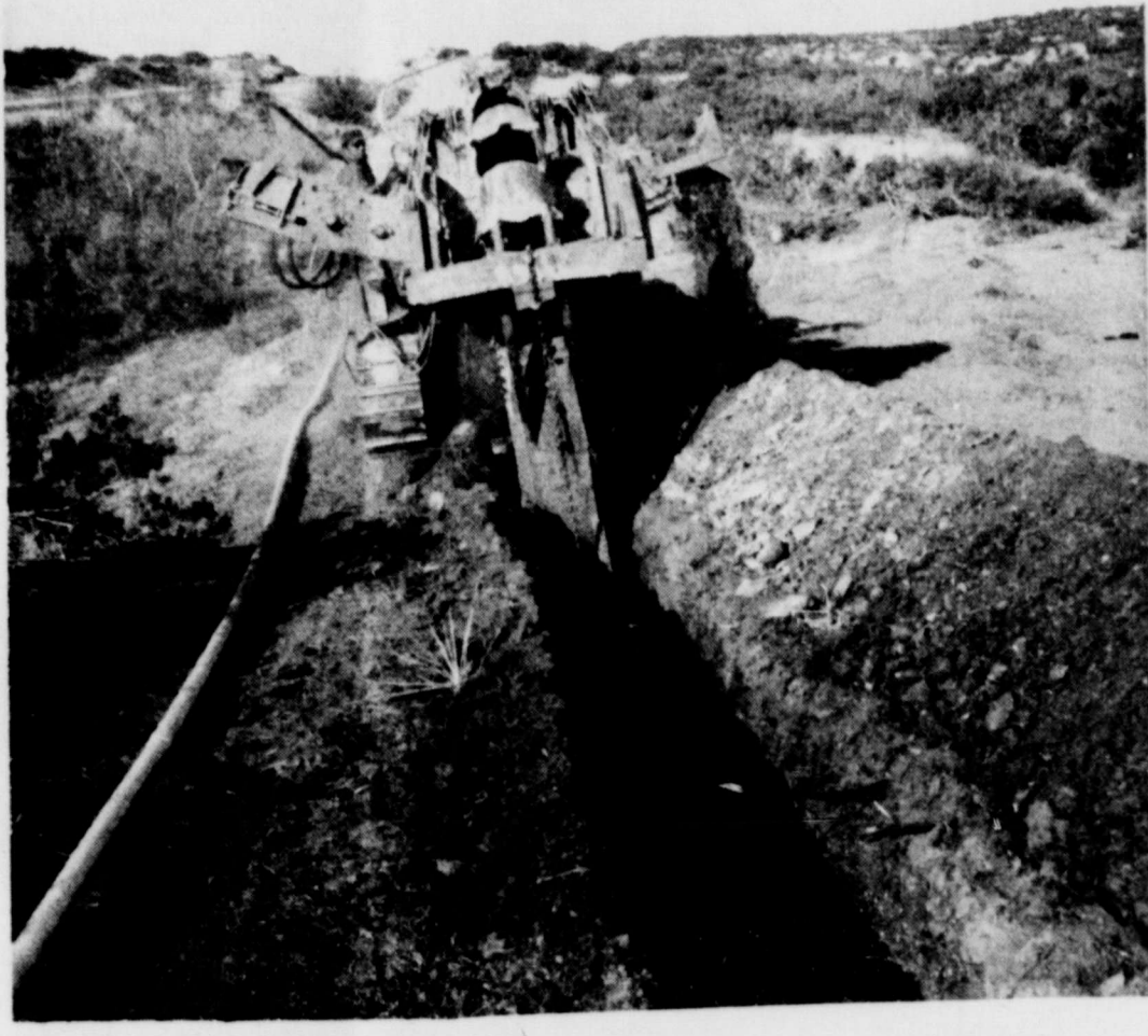
DITCHER AT WORK —This photo looks west to the top of the six mile hill west of Crowell as a Rhode Pipe Co. ditcher moves west. The white plastic water line is pictured to the left of the ditcher. A crew stays ahead of the ditcher putting the pipe joints together.
