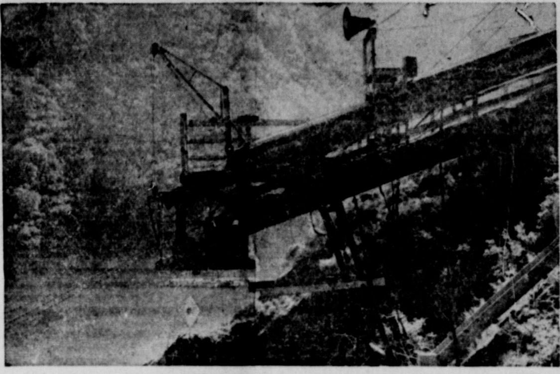
300-FOOT PEA-SHOOTER—FOR TORPEDOES... High in the fastness of California's Sierra Madre mountains the U.S. navy has developed and constructed what is probably the world's largest pea-shooter. Pictured above, the 300-foot tube, fired by compressed air, was built to launch naval torpedoes into Morris dam lake for exhaustive tests by naval ordnance underwater division experts. More torpedoes have been launched in this peaceful little lake than were fired by the Japanese during the entire course of World War II.
