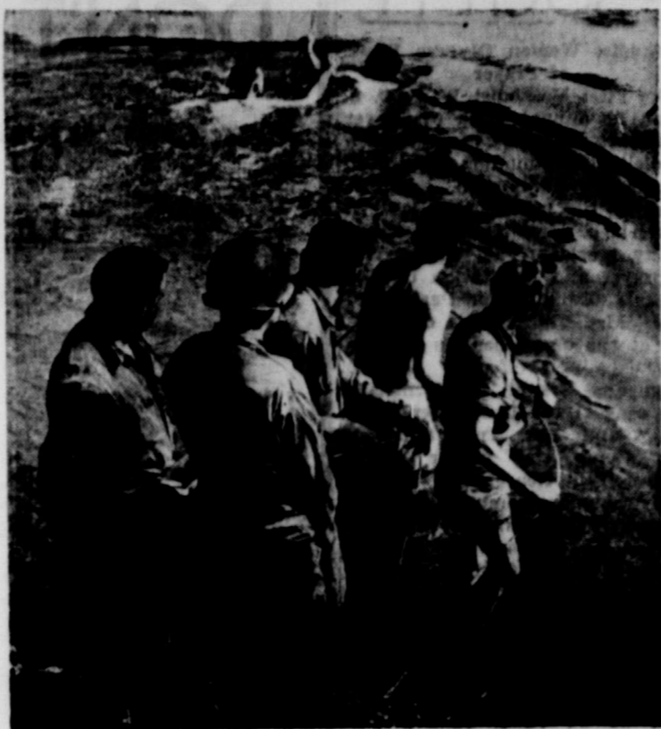
When communication lines laid across the Moselle river, France, by the signal corps batallion were broken three times, the men decided to swim the lines across the river. The signal corps work has been outstanding in this war in keeping open all lines of communication, many times under heavy fire.
