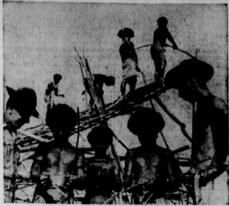
There is no timber in New Guinea, and so, when it comes to building, the American soldiers learn a trick or two from the natives near Port Moresby. Before the grass that is put on, the beams are securely tied with strips of bark which the natives are shown peeling. In the background the framework of one house is all but completed. Little forks that two of the natives wear in their hair are solely for pleasure—the pleasure of scratching.
