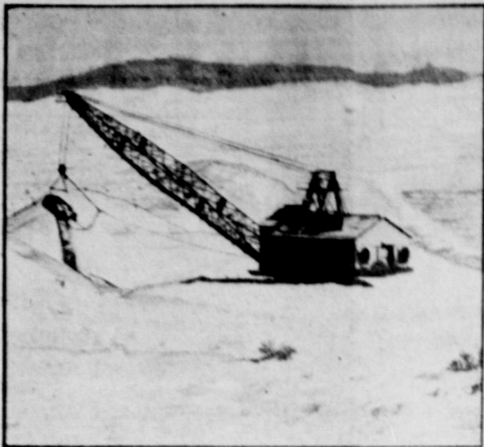
Across the snow white sands of the southern California desert, the Bureau of Reclamation is cutting America's greatest irrigation ditch, the All-American canal. Here a gigantic dragline is shown at work where the deepest cut, approximately 100 feet, is being made. The All-American canal will carry water from the Colorado river 80 miles over these wastes to the flourishing Imperial Valley. It follows closely the international boundary and will replace a canal which now extends 50 miles in Mexican territory.
