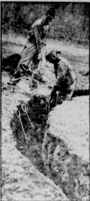
Embedded in concrete, the steel rods shown projecting from the pit will soon hold a strato balloon in leash, pending its ascent into the stratosphere. In the Black Hills near Rapid City, S. D., workmen are busy with preparations for the newest attempt, to take place within a few weeks.
