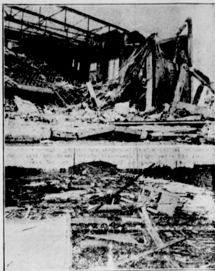
People who have never seen through a tropical hurricane cannot apprehend the ordeal endured by citizens of the Lower Texas valley, nor visualize the destruction of the building. Above is a picture of the municipal auditorium at Harlingen, showing great masses of concrete twisted and broken. Below the freight docks at McAllen are pictured in splinters.
