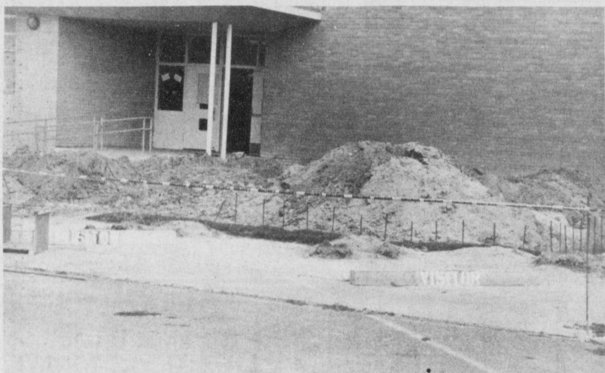
NEW LIBRARY FOR DILLMAN ELEMENTARY ---The foundation for the new library for Dillman Elementary School has been laid. The library will be located at the front of the school, next to the office. (Journal Photo)
