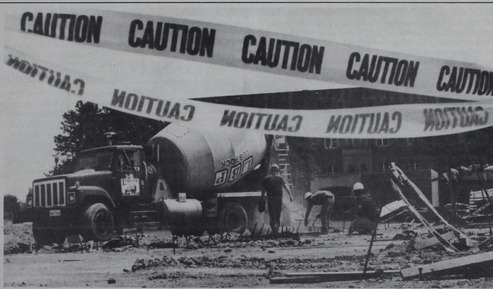
Brick by brick: Construction workers from Lee Lewis Construction Inc., work on the new Southwest Collection addition Tuesday afternoon. The construction for the new library was started Feb. 10 and is to be finished by late 1996.
