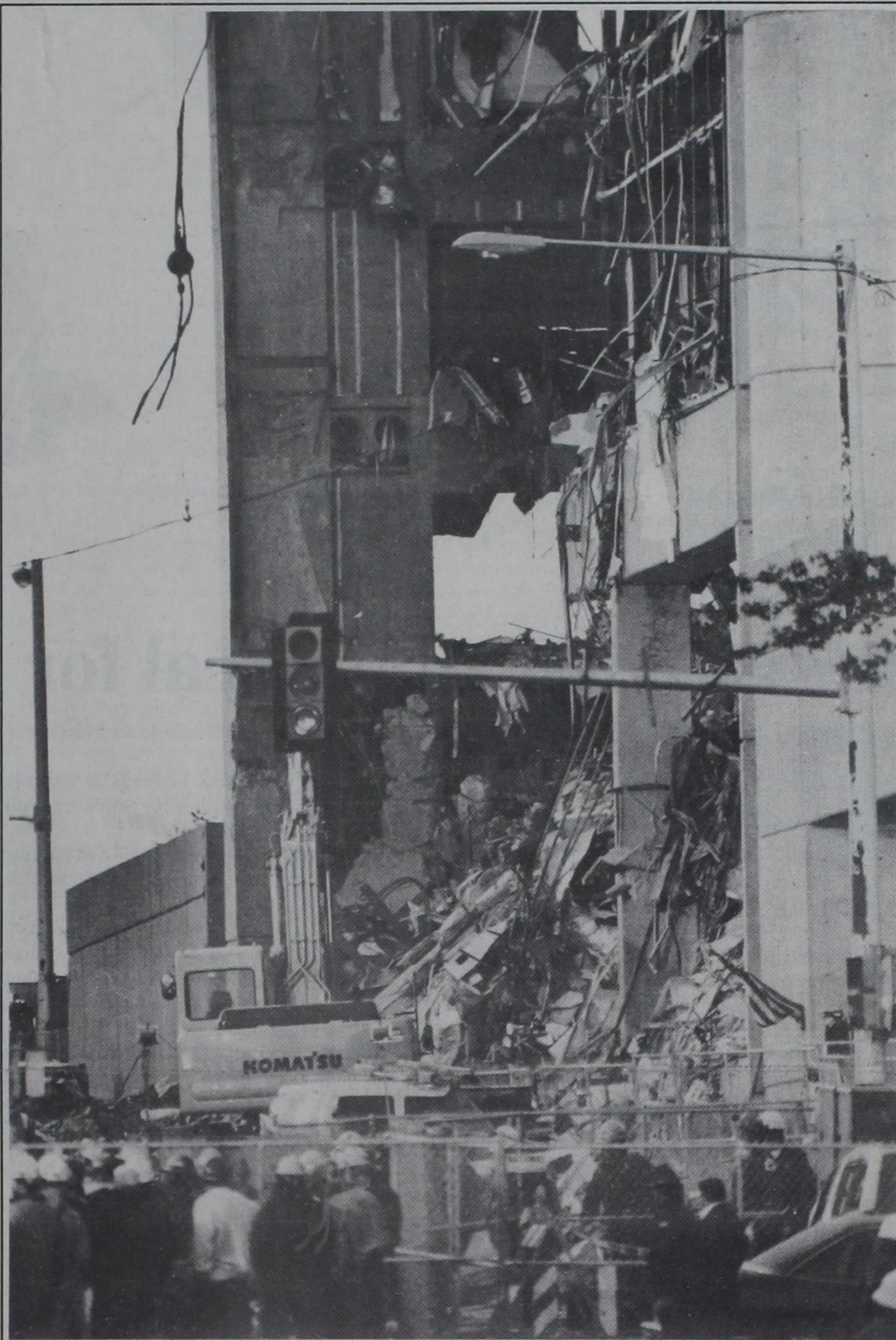
The search continues: Work crews gather early Thursday to prepare to shore up several weak sections of the Alfred P. Murrah Federal Building in Oklahoma City. Efforts to rescue victims trapped inside the building after Wednesday's bombing continue today.
