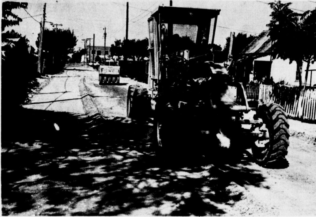
STREET WORK —Machinery begins preparing the surface of unpaved streets to receive the coats of primer and asphalt, in the current project to pave many of Winters' streets. The
