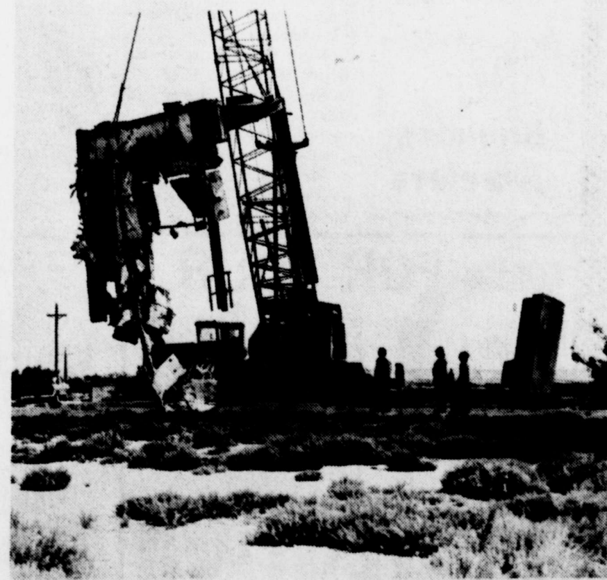
NON-HEROIC ENDING—The Atlas missile base about five miles east of Winters was, for a short time in the early Sixties, one of a network of defensive retaliatory space-weapon firing stations. In the deep underground silo rested, for a time, a supposedly, nuclear war-headed missile, kept ready for instant flight against an enemy. A close-guarded unit of the U. S. Air Force, the missile was manned and armed for only a few months, to public knowledge. For several years, the base has been
