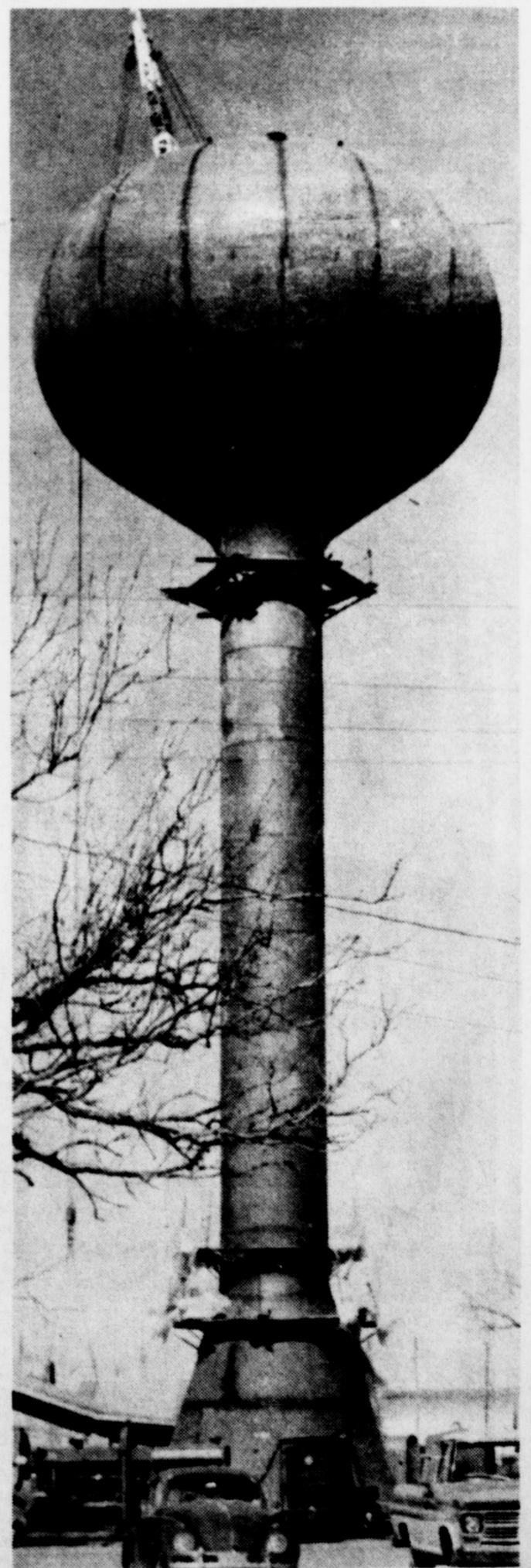
PROGRESS REPORT—The new water tower being constructed on North Main Street has the appearance of a giant golf ball on a tee, after workmen installed the huge ball on top of the tower. There still is much to be done before the storage tower is completed,
