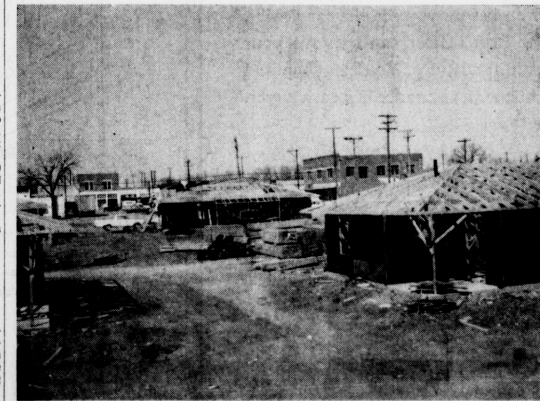
PROGRESS has been rapid on construction of the low-cost housing project for the elderly. Earlier photograph, taken from about the same spot and published January 28, showed only a few of the foundation and floor forms in place. Another section of this part of the project is located across the street north from this site. Excavations are being made and forms built for foundations and slab floors of the 16 units to be designated for low-income families, located in the northeast section of town.
