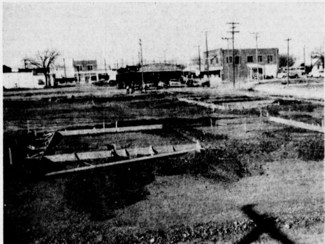
HOUSING — Forms were being built last week for foundations and flooring of some of the housing units in the project of the Winters Housing Authority. Units which will be constructed on sites shown here are located on East Parsonage and Grant streets, and will be for the elderly. Other units for this part of the project will be located north of East Parsonage. Work also is being done on the part of the project located in the northeast section of town near the schools, which will be designated for low-income families. (Staff Photo)
