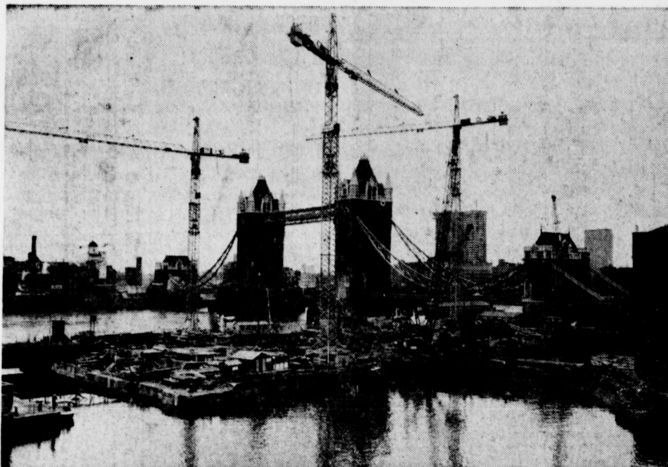
GIANT CRANES dwarf London's Tower Bridge as St. Katherine Locks redevelopment scheme gets under way. Project will provide London with its first yacht basin, housing for 650 families, three schools, an entertainment complex, a chapel, sports center and an 830-room Tower Bridge hotel upon expected completion in 1973.
