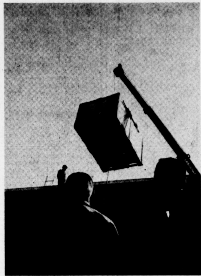
SKYHOOK!—M. D. Johnston, left, and the Rev. Harry Grantz, pastor of Winters First Baptist Church, watch as workmen hoist one of two heating-refrigeration units to the roof of the church's educational building. The units provide heat and refrigerated air conditioning to the building. (Staff photo)
