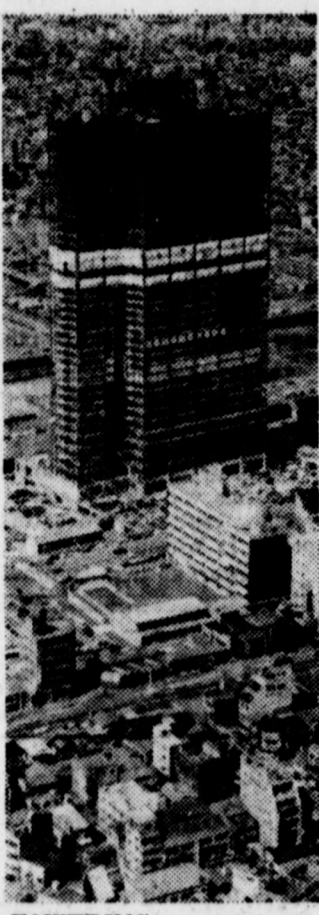
TOWERING over everything for miles around is the framework for a 44-story Tokyo hotel which, when completed, will contain 1,057 rooms and cost more than $36 million.
