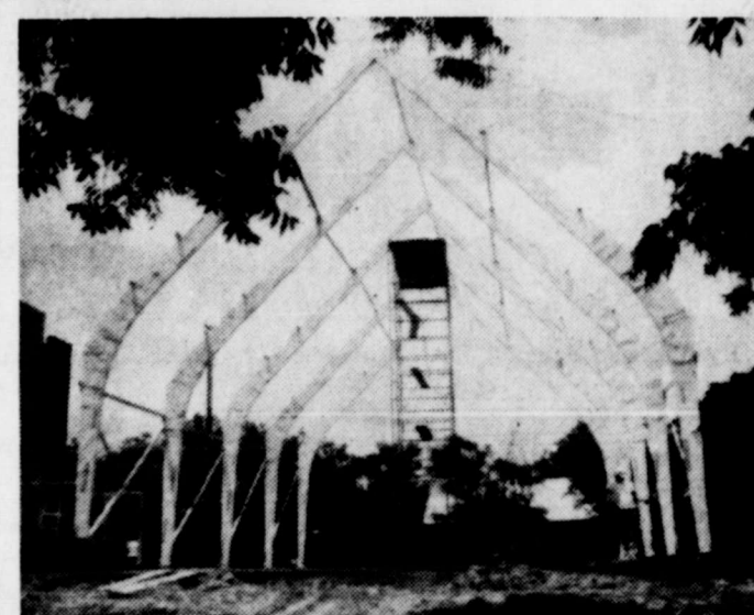
SHAPE OF THINGS TO COME: Resembling giant whale bones, the roof and wall girders of the new United Methodist Church sanctuary rise against a cloud-dotted May sky as the new church building takes shape. The big girders, made of laminated yellow pine, weigh about 1800 pounds — for each "rib"—and
