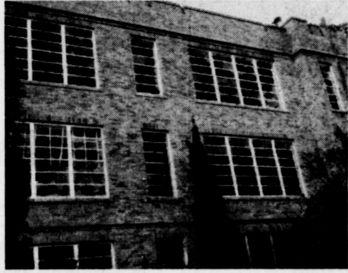
HIGH SCHOOL —Every window on the front of the Winters High School was broken out by the hail. All buildings of the school plant were damaged, and
