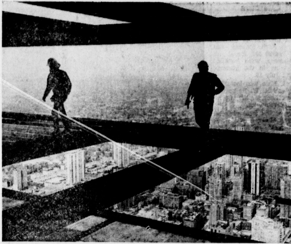
STROLLING along beams on the 90th floor of the 100-story John Hancock Center, workmen are silhouetted against a backdrop of Chicago's north side. When completed, the 1,431-foot structure will be world's second tallest skyscraper.
